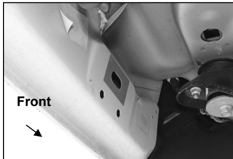
(Fig 1) 2009-mid 2015 Driver/Left front mounting location (No factory holes in pinch weld 2009-2011 models)
