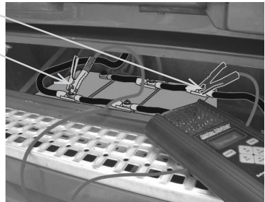
Battery Bank of 3 Batteries
