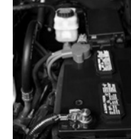
Battery without corrosion
