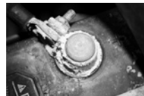
Corroded Cable Connection
