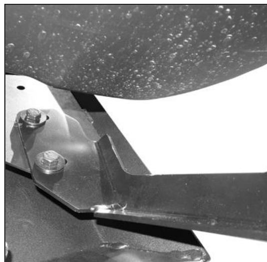
(Fig 11) Passenger/Right Side complete installation
