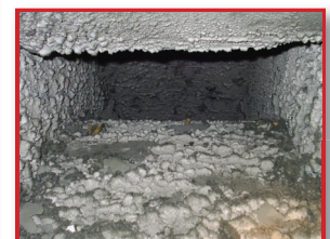
A probe's-eye view of a filthy air-conditioning duct
