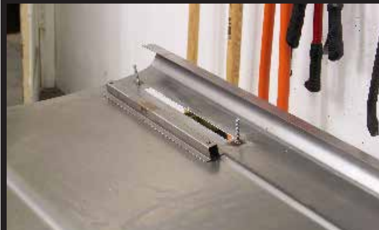
6. Weld two bolts to the inside of the combo skin that lines up with the holes in the U-bracket.
