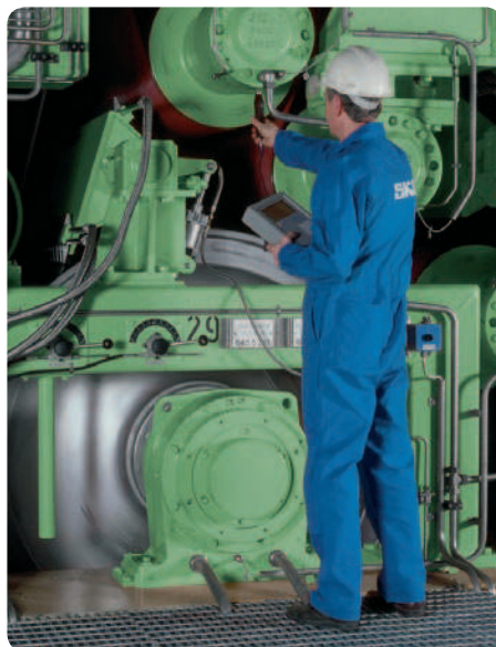
Checking vibration levels
