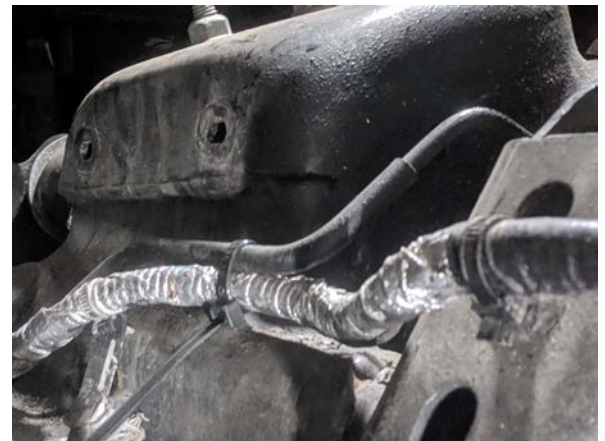
Detail 20b: Wiring secured to brake line
