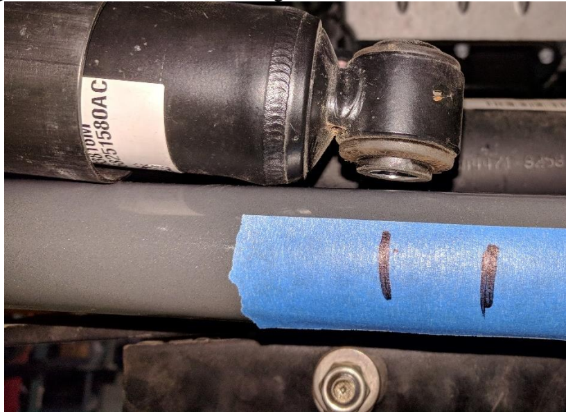
Figure 3. Steering Turned Full Passenger, Stabilizer Collapsed
